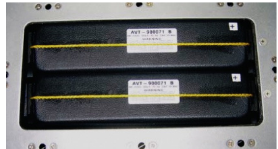
Cover removed, exposing 2 Lithium Ion batteries
