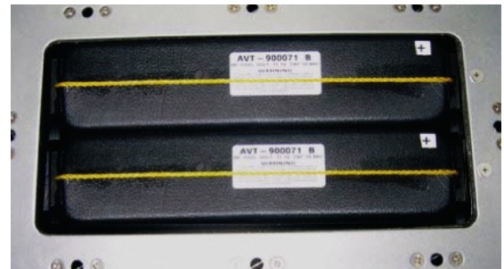
Cover removed, exposing 2 Lithium Ion batteries
