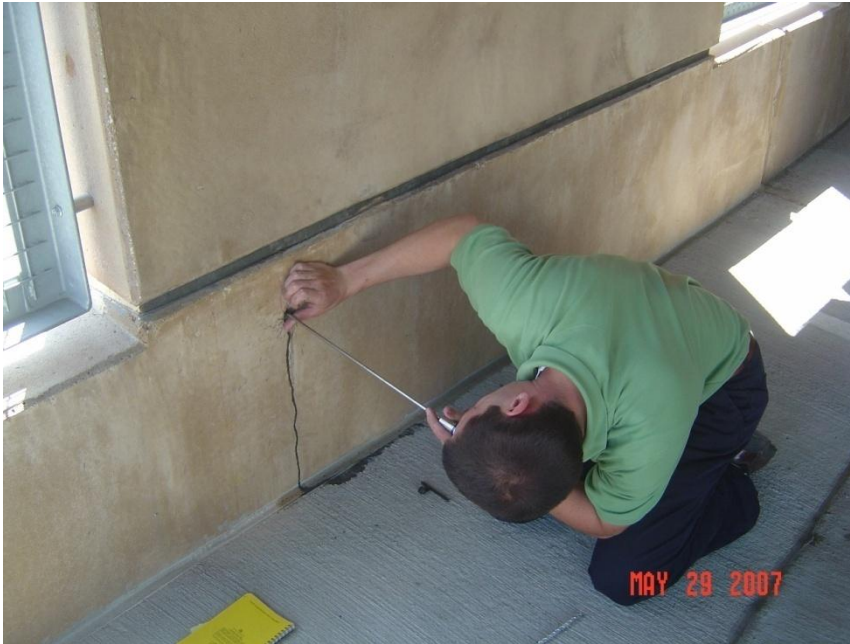
Figure 13- View of an exploratory opening at a voided splice sleeve
