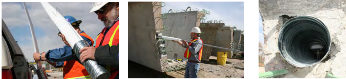
Figure 3 – Styrofoam supported by wire rod (left), the foam rod being inserted into the duct to form voids (center) and view of Styrofoam defect inside a duct (right)
