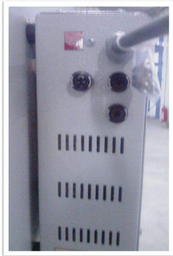
Picture 2: The Rear Section of the Control Box
